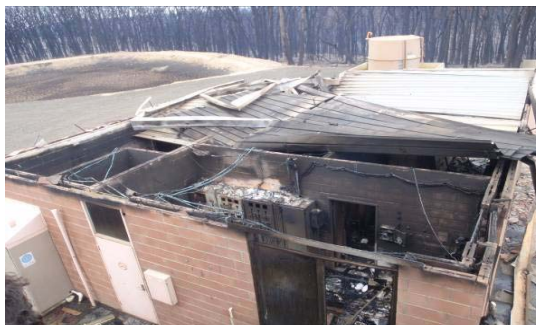
Figure 1: Burnt out dosing and control room
