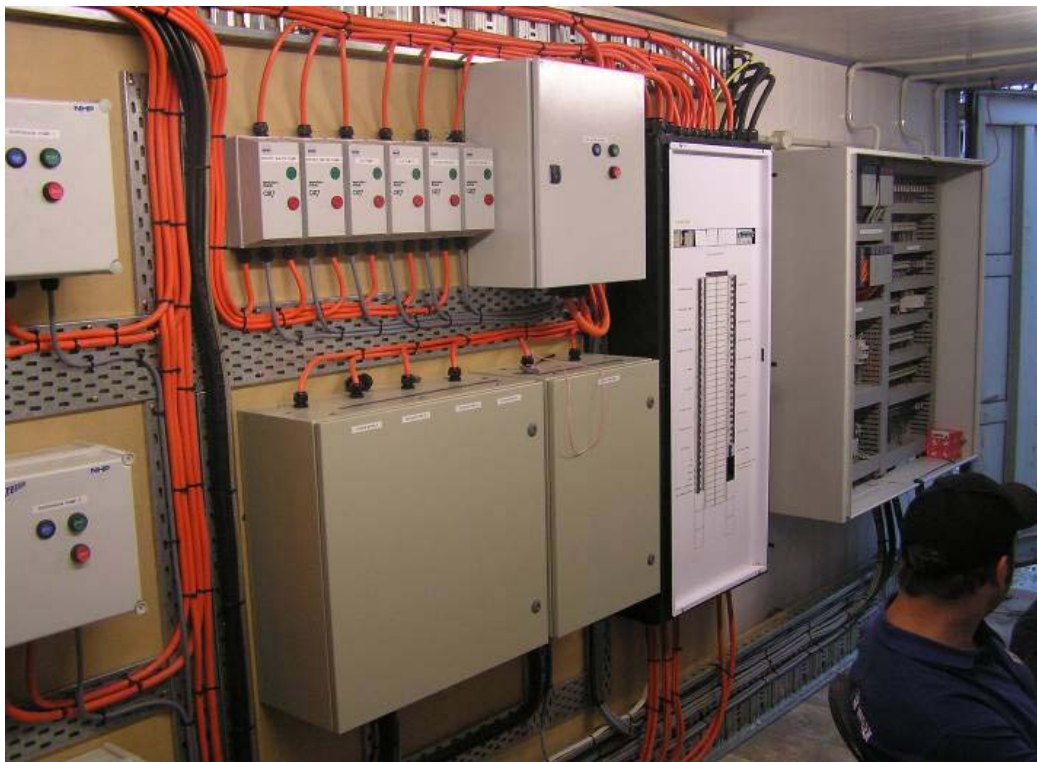
Figure 4: The finished control room
