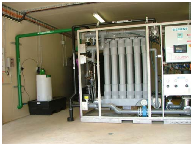
Figure 2: Girgarre membrane filtration unit
