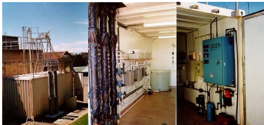
Figure 3: Ozone Pilot Plant
