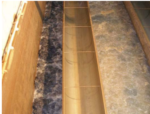
Figure 1: Kyabram filter in air scour
