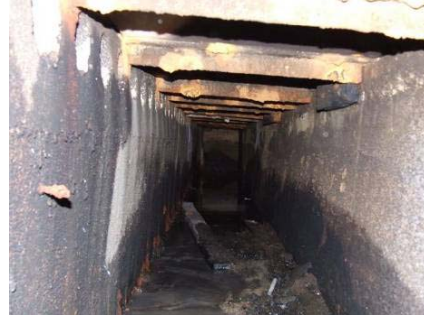
Figure 4: Rubbish in the plenum trough
