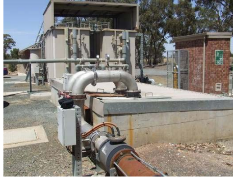
Figure 7: The low level of the roof and open end were retro fitted to improve entry to filters and wind holding back float.
