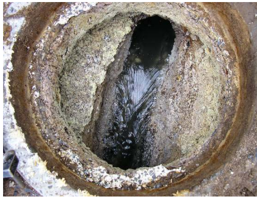
Figure 1: Concrete ‘Corrosion’ Within Sewer Manhole
