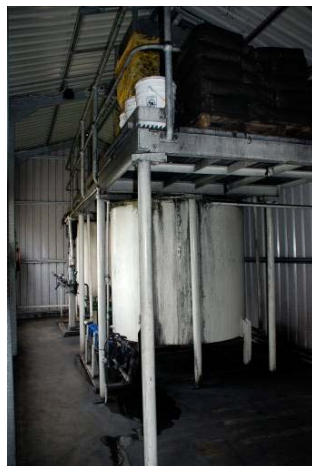
Figure 4: PAC Dosing Equipment
