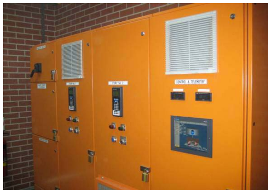
Figure 3: Transfer Pumping Station switchboard fitted with touch screen
