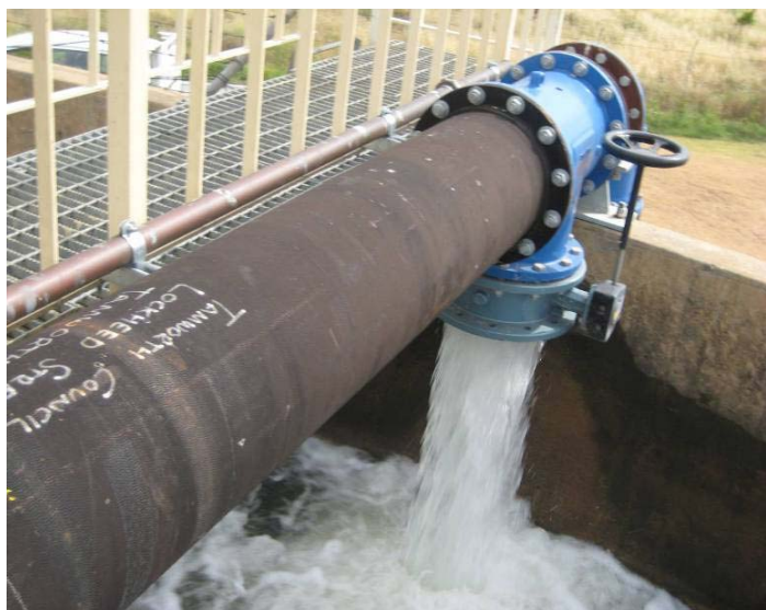
Figure 6: Well water pumping into raw water tank at Water Treatment Plant
