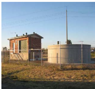
Figure 4: New Pump Station and Balance Tank
