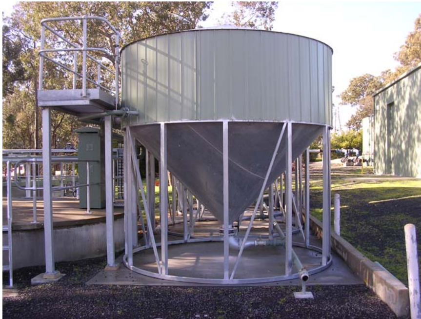
Figure 5: Secondary Sludge Silo
