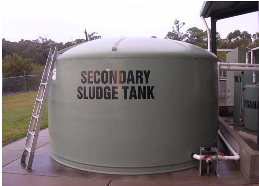
Figure 4: Secondary Sludge Tank
