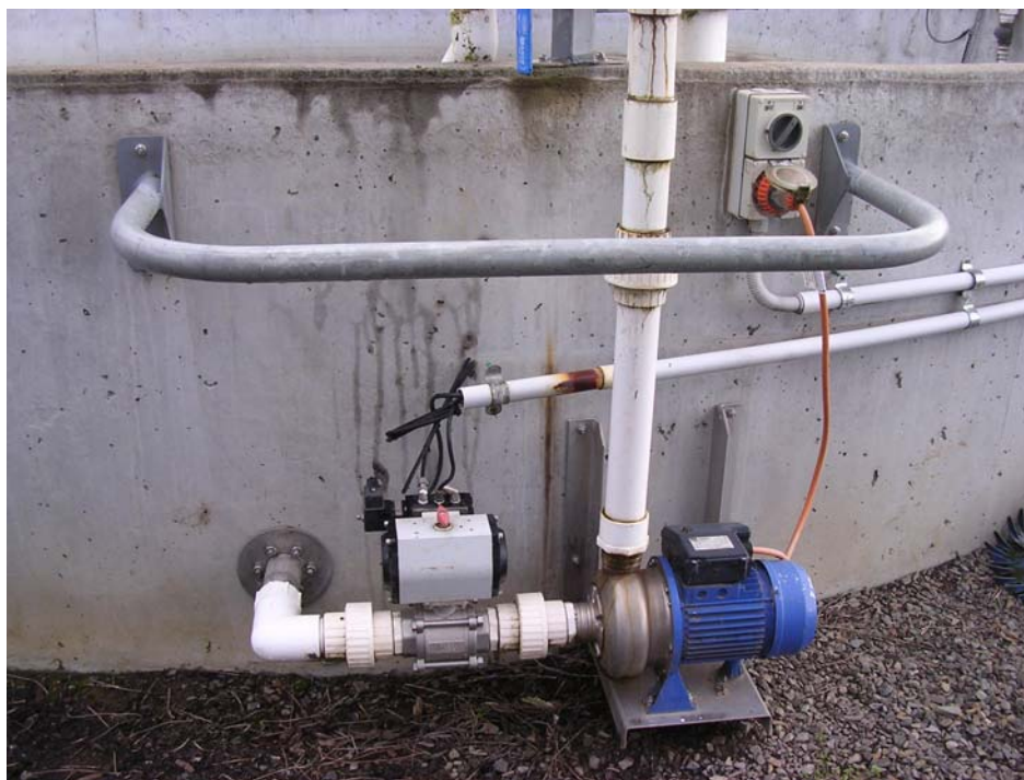
Figure 3: External pump configuration
