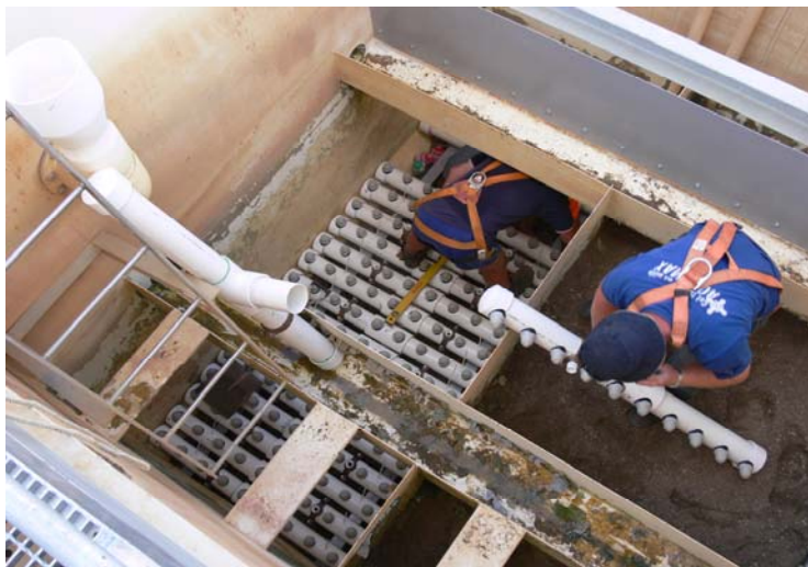
Figure 1: Installation of ‘hungry boards’ to backwash troughs and 100 NB uPVC Class PN 18 nozzle pipes to the underdrain system
