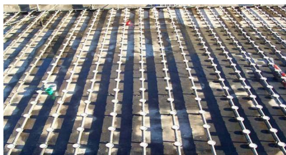
Figure 5: Diffuser in Bioreactor #1
