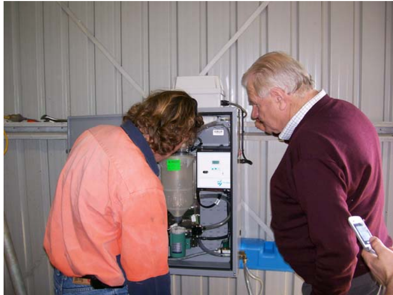
Figure 1: Chemsearch’s Peter Bennett explaining the operation of the Bioamp to Council Treatment Plant operator Marcus O’Reilly. The Bioamp installed inside inlet screen room at The Dru Point Wastewater lagoons 13/10/07
