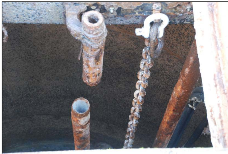
Figure 2: Badly corroded pump guiderails
