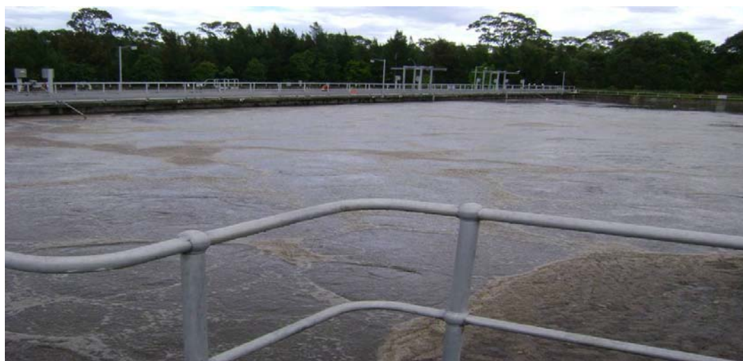
Figure 3: Bioreactor #2 at the Edgeworth WWTW
