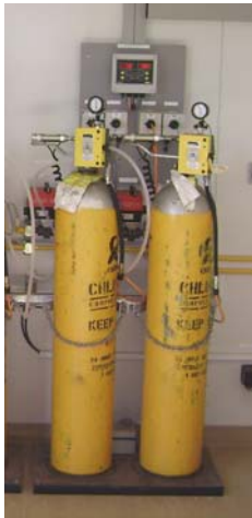
Figure 1: Chlorine cylinder storage
