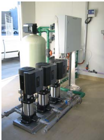
Figure 12: Pressure pump set & sand filter
