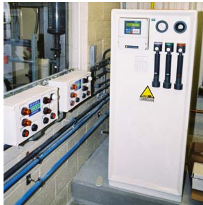
Figure 8: Onsite sodium hypochlorite generator
