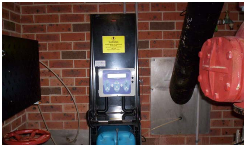
Figure 3: Portachlor Hypochlorite dosing system
