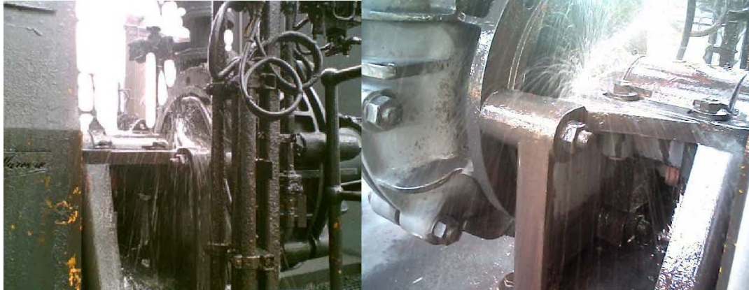
Figure 2: Examples of excessive leakage to atmosphere
