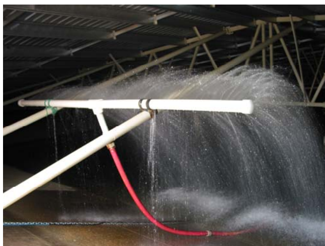
Figure 2: Aeration at Denmark Horsley Road Reservoir
