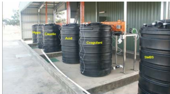
Figure 2: WRP Chemical Storage Area
