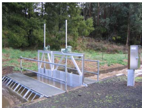
East Barwon River Automated Channel Gates Controlling Floodwaters into Channel during flood
