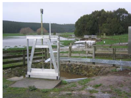
Pennyroyal Creek Automated Channel and Diversion Weir Gates
