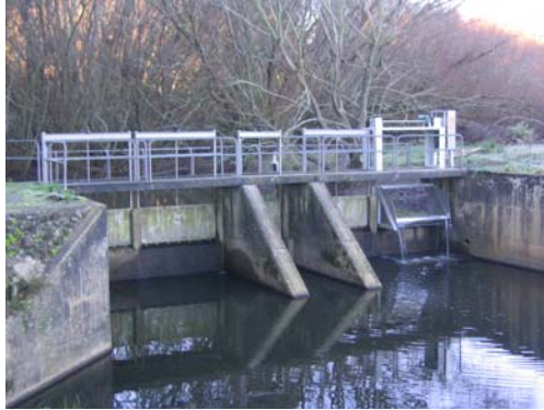
Automated gate right of picture at Callahans Creek Diversion
