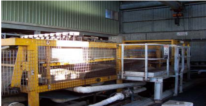
Figure 5: Existing Filter Belt Presses
