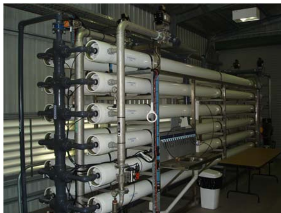
Figure 5: Membrane Vessels – The Basis of Reverse Osmosis
